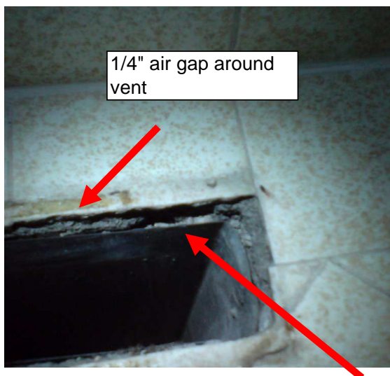
air supply vent leakage
