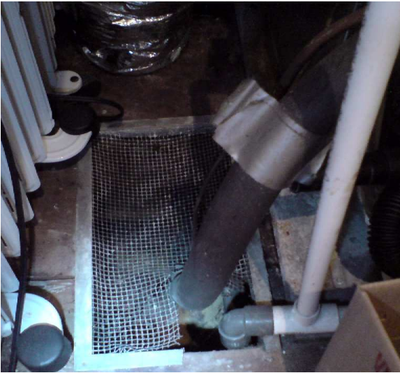
inside furnace closet, large hole open to dirt crawlspace
