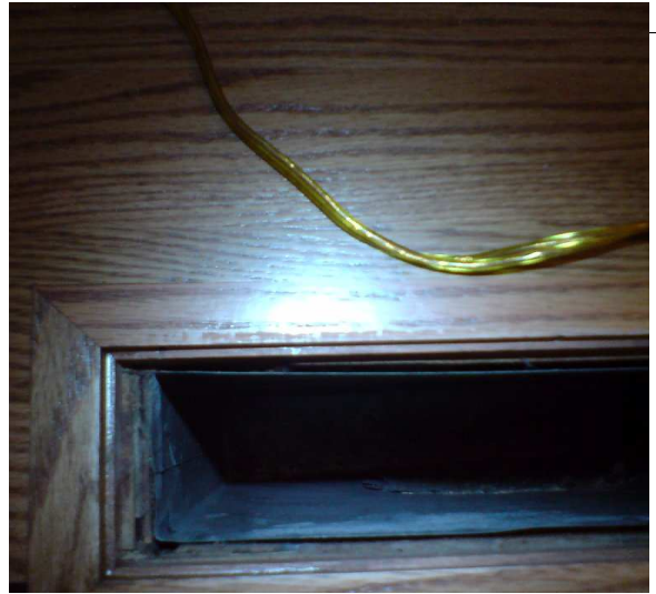
air supply vent leakage, seal leaks
