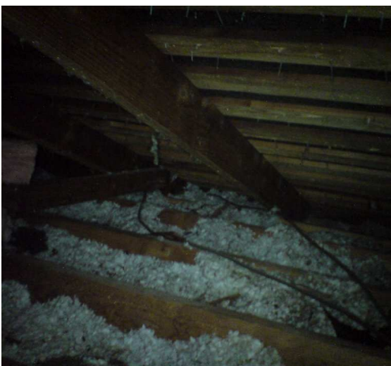
existing attic - no barrier
