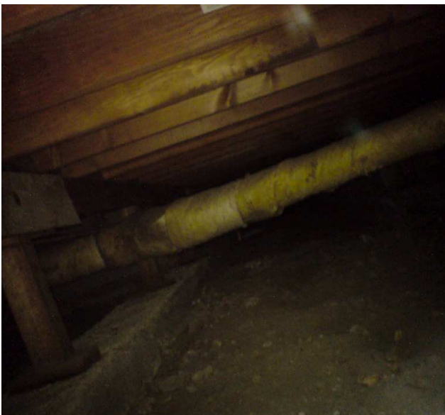
photo of home's ducting, wrapped in fiberglass; notice dark dust spots
